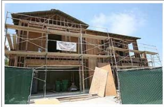
This and other Ocean Heights subdivision homes are in the process of being rebuilt due to severe rain damage and mold. Owners are suing the builders for the the cost of the poor construction.
